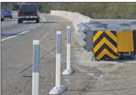
Impact attenuation protection
