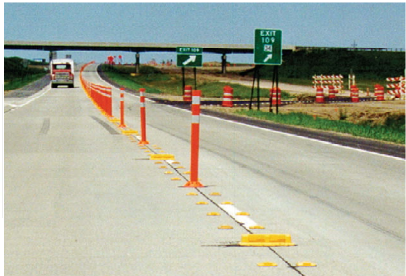
The Brick, the RPM and FG300 in a typical 2-way 2-lane detour
